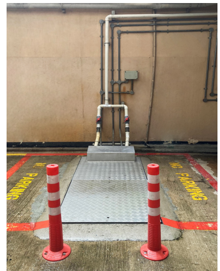
Water storage tank for groundwater harvesting
